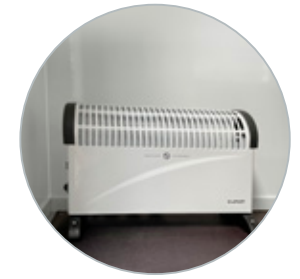
Electric heating (1500 Wh) in accommodation space
